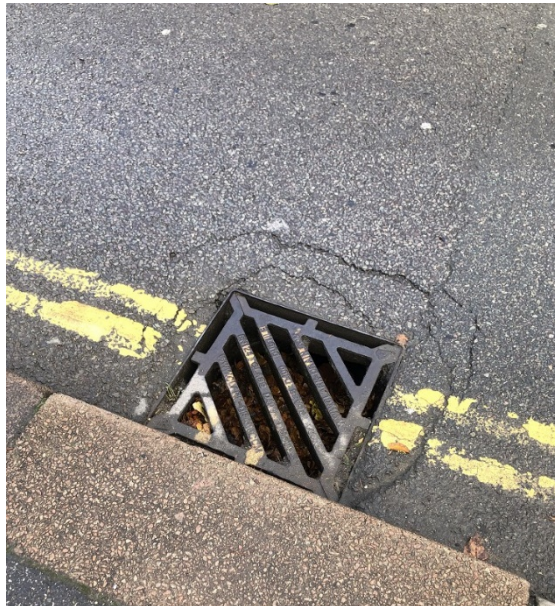
Image 5 – Carriageway defects surrounding partially blocked gully west of crossing (south side of B1042)
