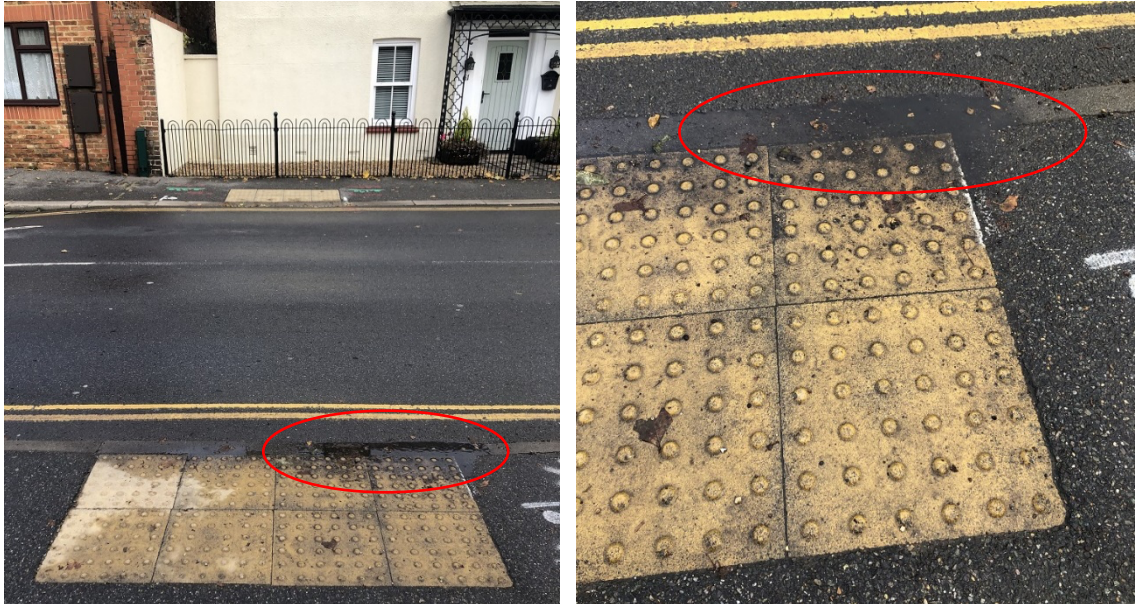
Images 1 & 2 – Evidence of surface deposits and ponding
